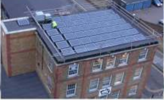
view of the solar panels from Craik Court
